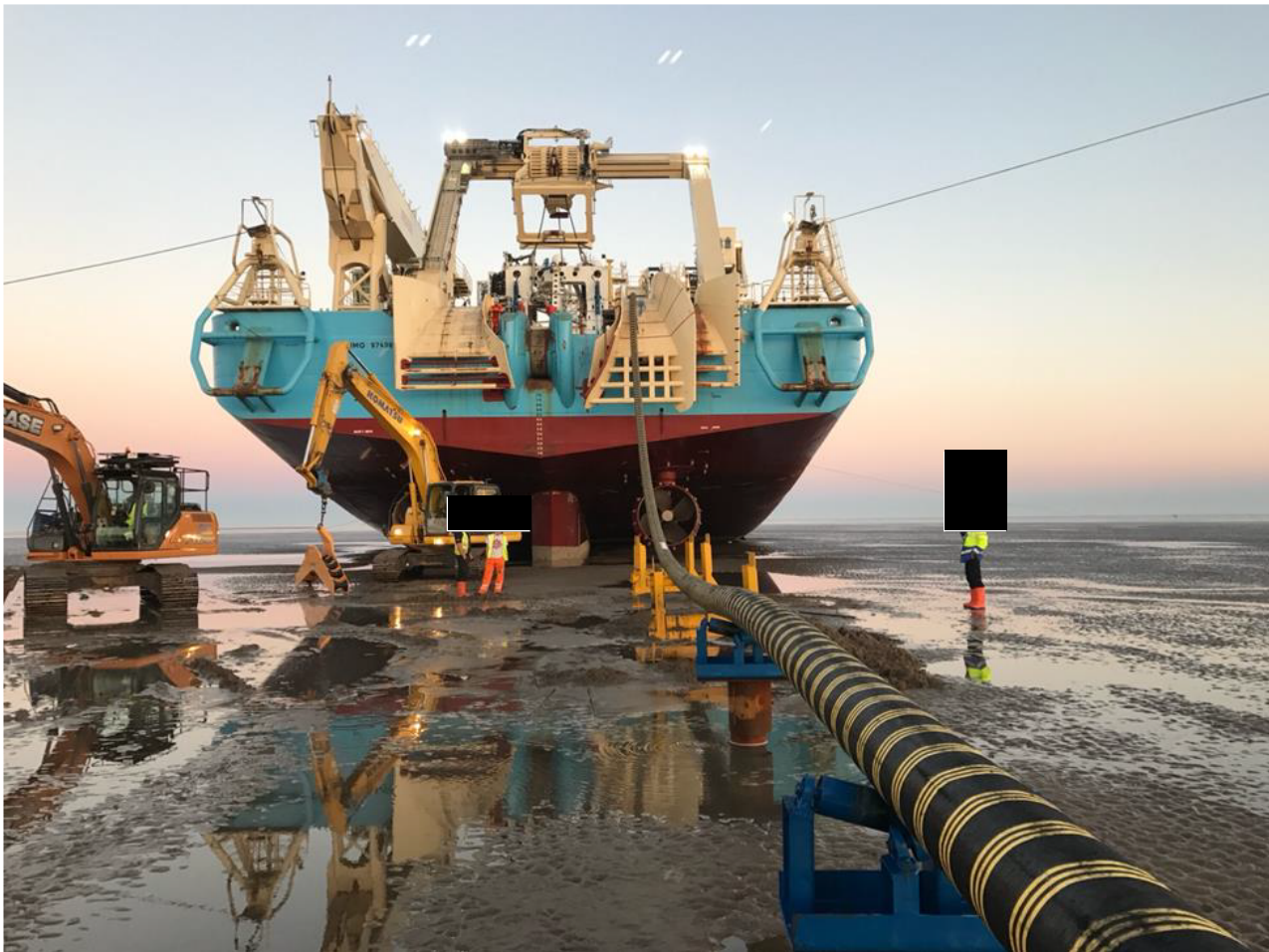
Plate 4.2 Example of cable being pulled ashore from a beached CLB (Walney Extension Offshore Wind Farm)
